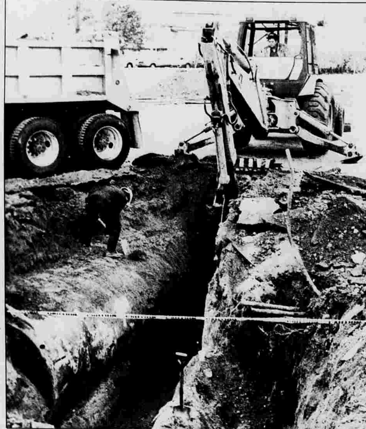
UNDERGROUND LABOR — Bruce DeVanney of Marlborough operates a backhoe while John Zaine Jr. of North Windham clears dirt around an underground gas line Friday at Manchester Police Headquarters. 239 E. Middle Turnpike. The two, who work for Casson-Matava Corp. of 53 Slater St., were preparing to remove the tank to comply with state laws requiring the replacement of tanks which are 20 years old or older.
